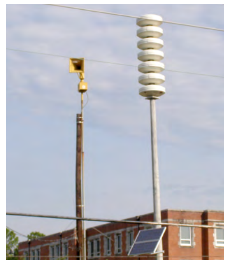
An old warning siren (l) that has been replaced by a new solar-powered siren (r).
