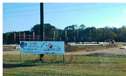
Construction began on the Polk's Meat Products processing plant in Simpson County Industrial Park in Magee.
