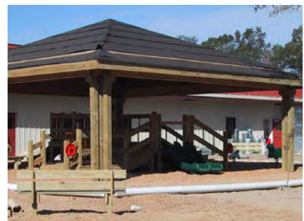
Construction of the Wee Care Child Care Center, funded in part by a loan from CMDC.
