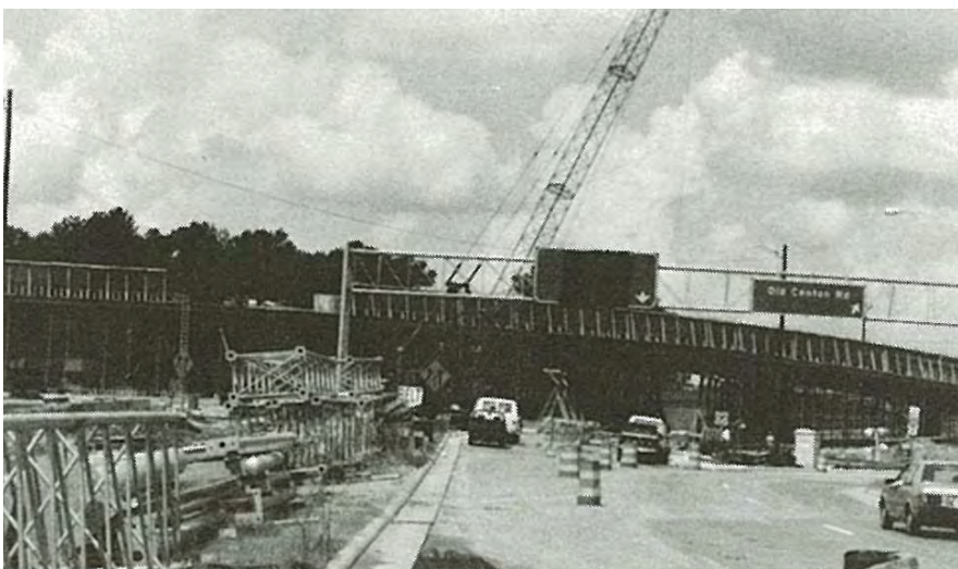
Photos show progress in construction of the Old Canton Road overpass on I-55.
